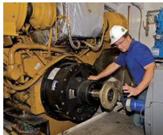
Project Manager Rick McKenna explains how one of the Campbell’s electric motor-generators, right, is connected to the starboard main engine, left, with a clutch, covered by black housing.
