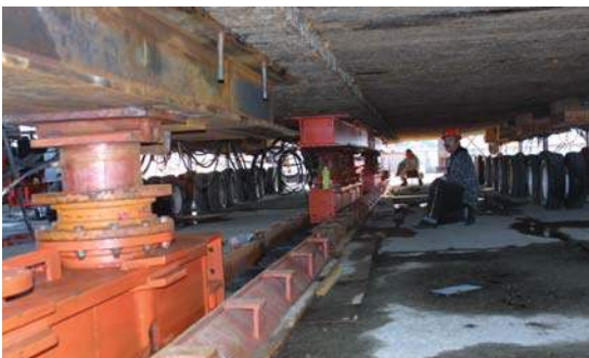
The drydock was mounted on 16 jacks, each with eight wheels, and towed from the barge to Foss Terminal. Ron Becker monitors the towing mechanism.
