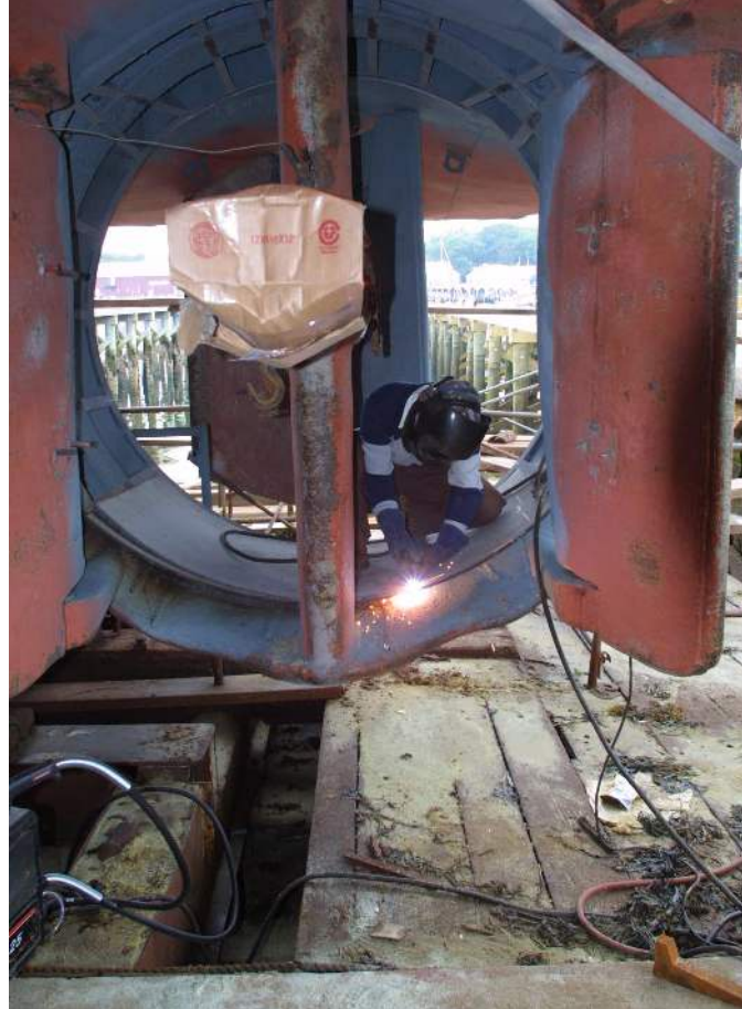
Foss Shipyard Welder Thin Tien Nguyen repairs the kort nozzle on one of Constellation’s tugs. He and another Seattle welder traveled to Gloucester, Mass., to perform the work.
