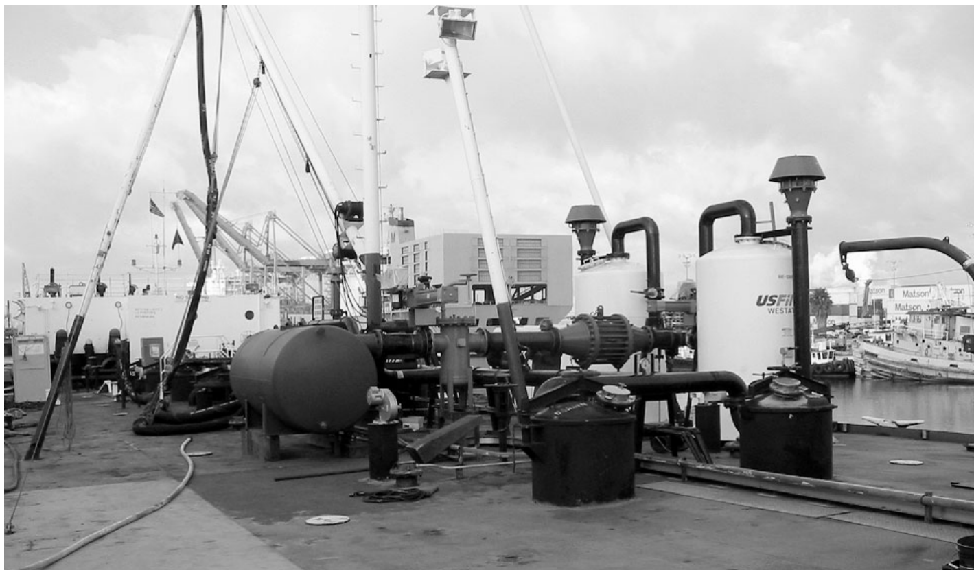
The tankbarge San Pedro is now equipped to process vapors displaced when tankers load cargo.
