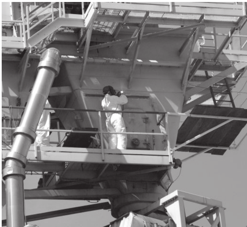
A welder works high in the superstructure of the Kivalina at Foss Shipyard, preparing the lightering barge for Foss' 15 th Season at Red Dog Mine.
