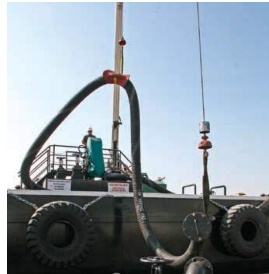
Joe Sasso uses the barge's crane to line up its product hose with a supply line at an oil terminal at the Port of Los Angeles.
