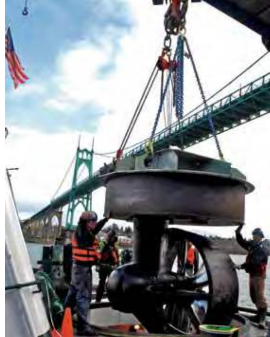
Workers at Advanced American Construction install a rebuilt Z-Drive in the tug PJ Brix . The tug remained in the water for the job.
