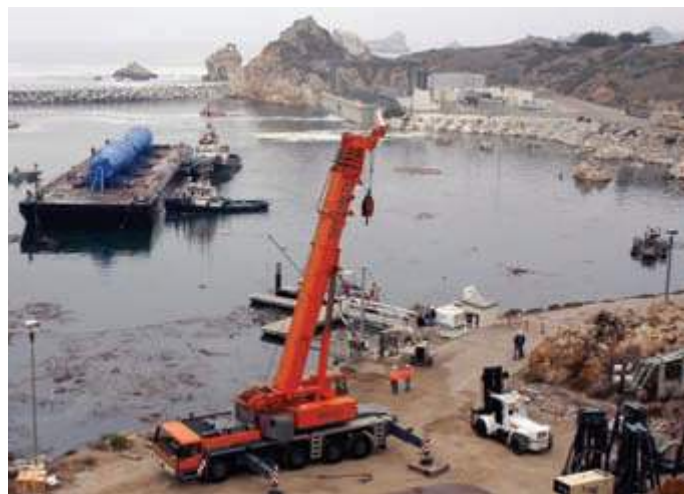
Two Pacific Tugboat vessels bring the barge ZB-240, which they have just received from the Foss Tug Howard Olsen , into the inner cove at the Diablo Canyon Nuclear plant.
