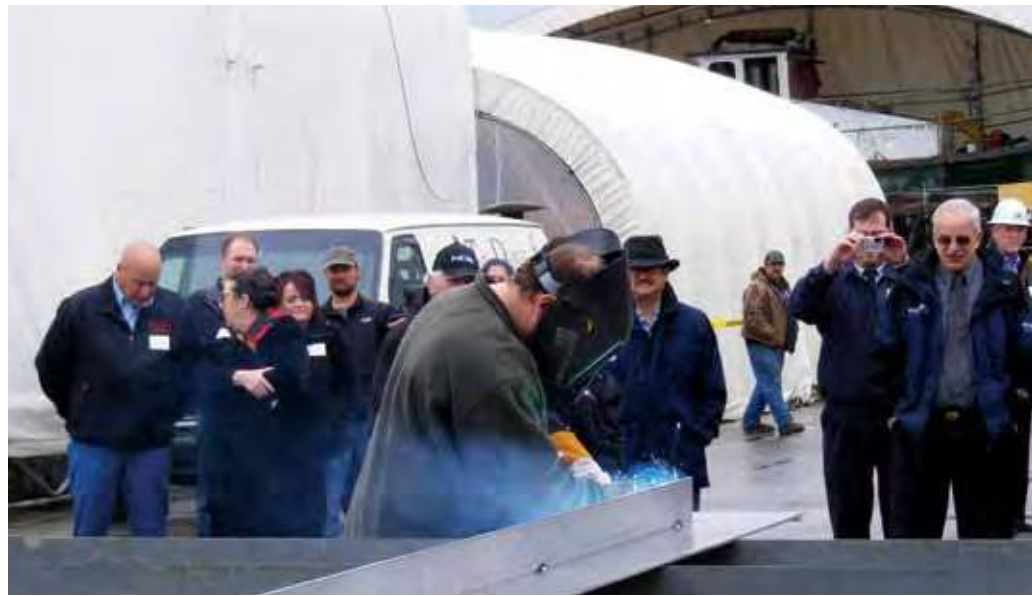
Keith Gorans welds a representation of the ferry's vertical keel onto an aluminum plate at the keel-laying ceremony.
