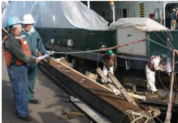
Shipyards Health and Safety Coordinator Ron Sykes , right foreground, and shipwright Mark Inabnit conduct an observation of welding operations on the Washington state ferry Rhododendron as part of the company's behavioral safety program.
