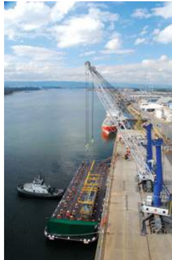
The Pacific Escort stands by as two big Liebherr cranes lift the first module onto the specialized barge Foss 286-3.
