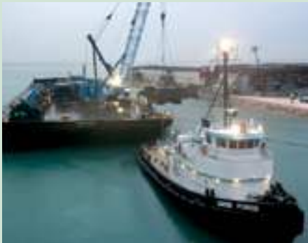
The Caribe Pioneer stands by as a lower section of the crane is hoisted onto the barge Columbia Boston .
