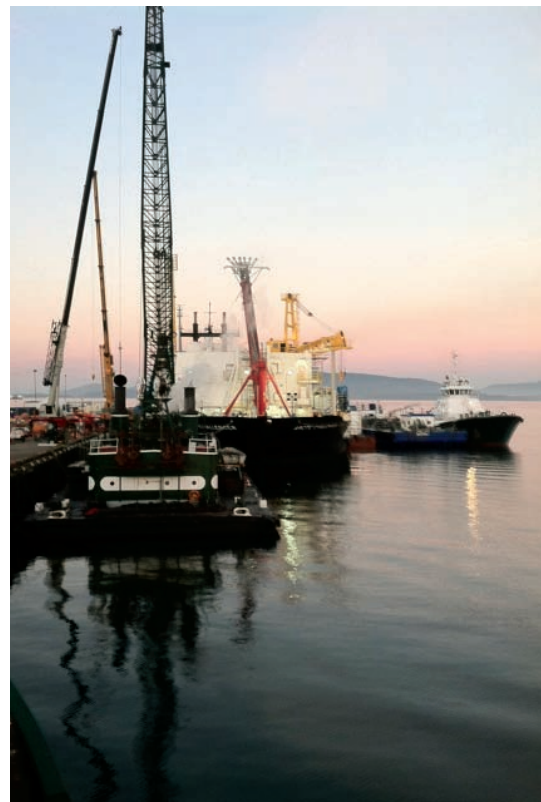
The Foss 300 derrick loaded materials onto the oil-containment barge Arctic Challenger in early September, while the Lindsey Foss , right, provided assistance. The photo was taken from the Corbin Foss , also assigned to the project.
