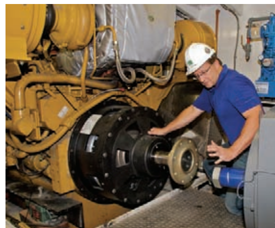
Project Manager Rick McKenna explains how one of the Campbell ’s electric motor-generators, right, is connected to the starboard main engine, left, with a clutch, covered by black housing.
