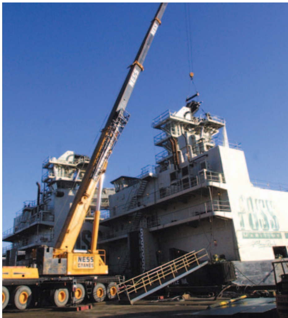
A Ness crane lowers a new "pocket belt" into position at the top of the elevator tower of the lightening barge Noatak . The belt distributes ore to the barge's boom conveyor system.
