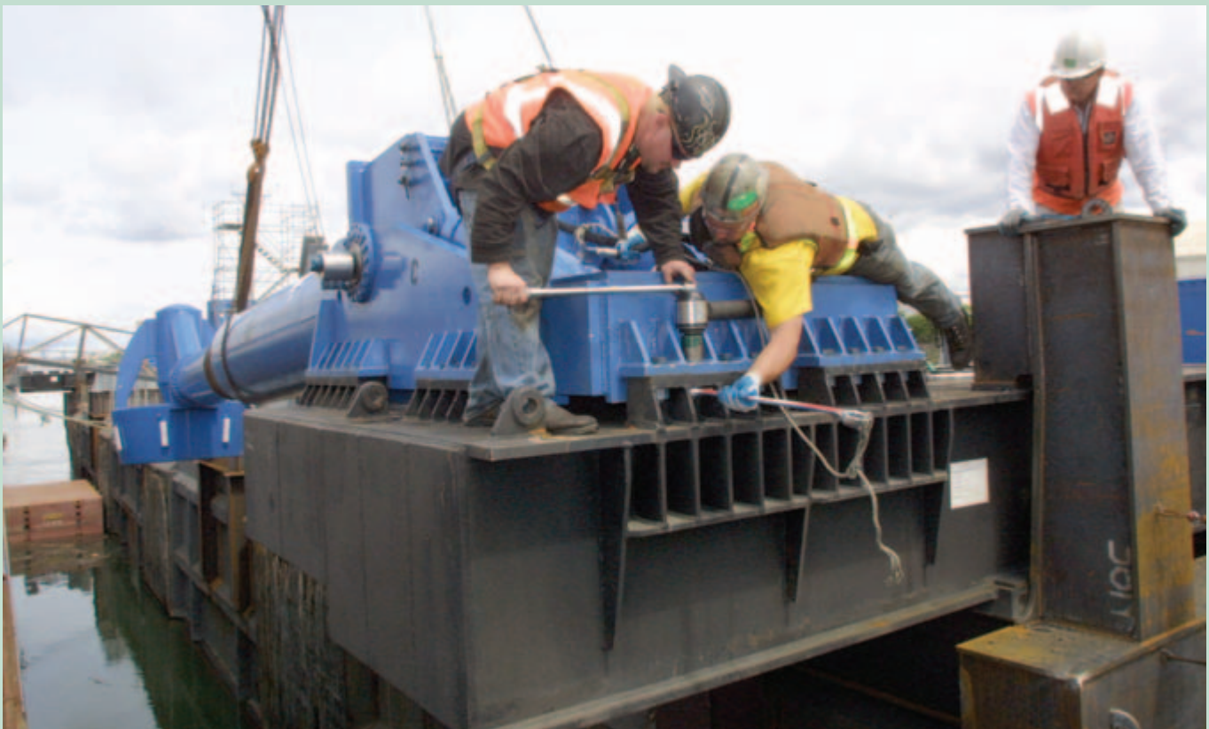
Foss Shipyard Machinist Gino Aiello , left, torques a bolt holding one of four 31,000-pound, 30-foot-long thrusters to the barge Marmac 12 . The thrusters will maintain the barge's position as it serves as a lifting platform for roadway sections of the new Tacoma Narrows Bridge. Holding the nut in place is Terry Dawley , rigger. At right is Superintendent Greg Schaut .
