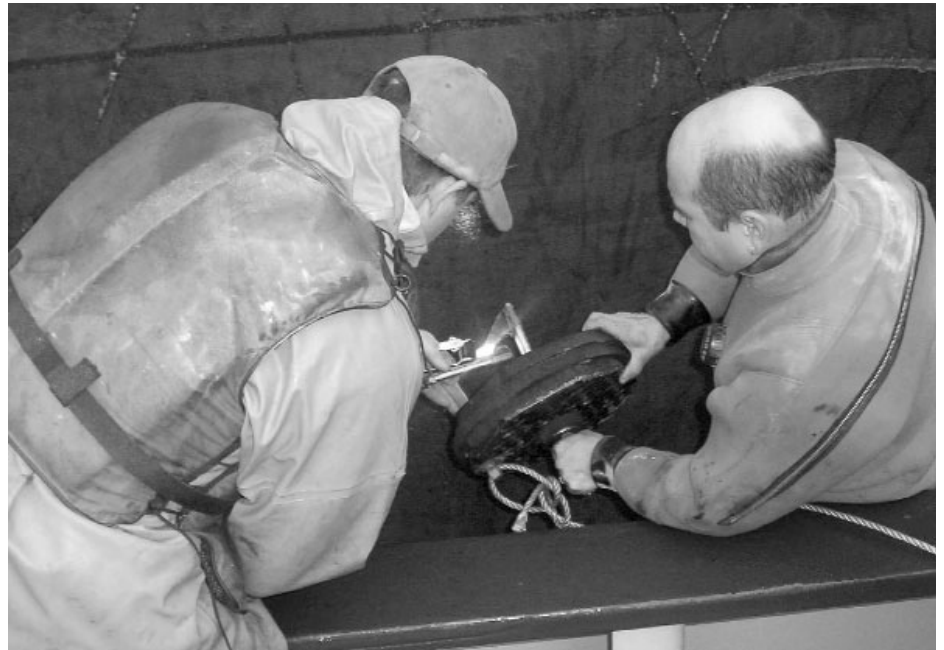
Salvage crew members Scott Miller , left, and Tom Ohryn prepare to apply a patch, fabricated aboard the Lauren Foss , to a freighter off the coast of Washington.
