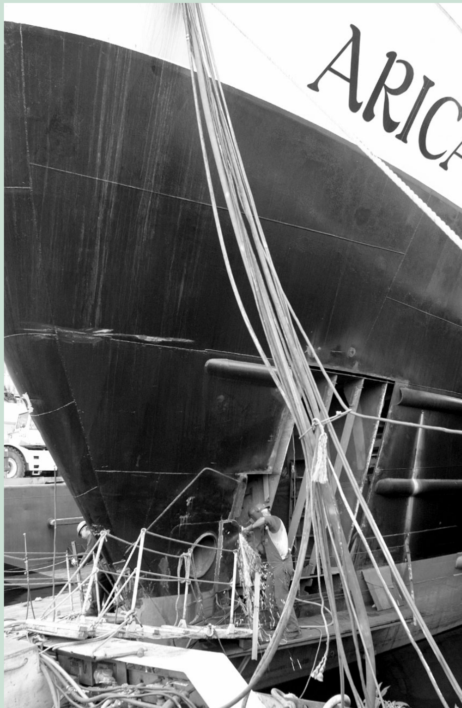
Replacing steel in the bow was among jobs performed this fall on the trawler Arica at Foss Shipyard.
