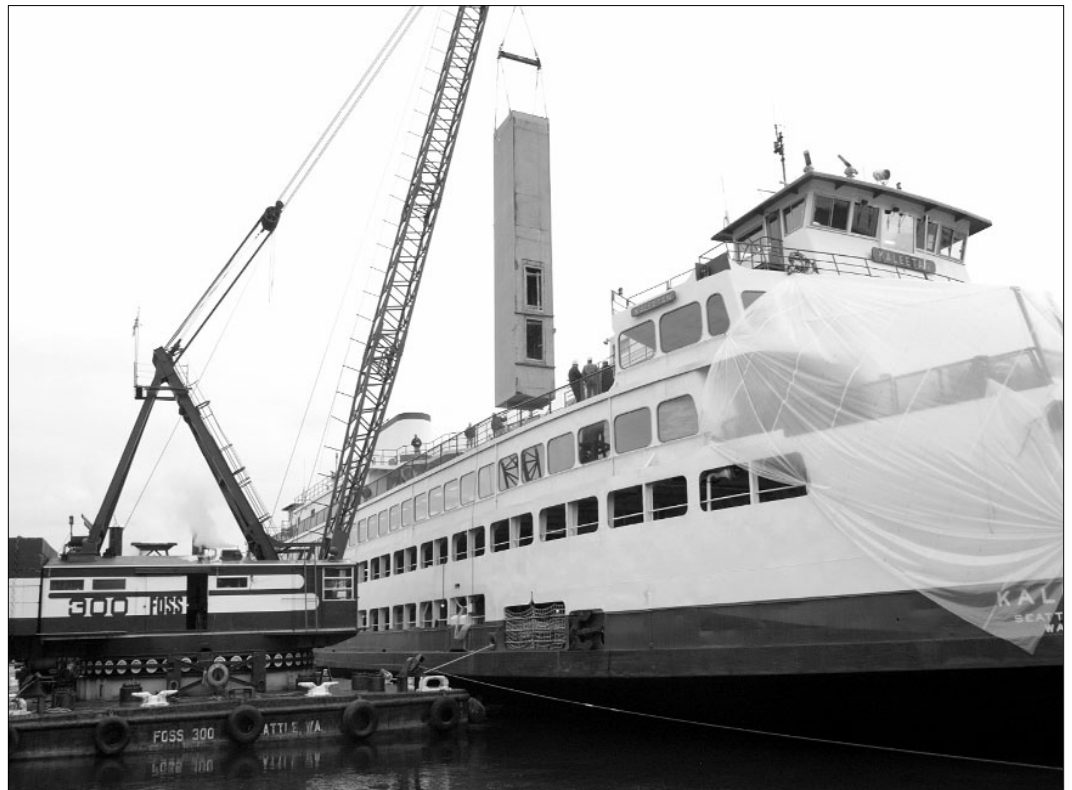
The steam derrick Foss 300 lowers a 47-foot-long, 33,000-pound elevator shaft into the Washington state ferry Kaleetan.
