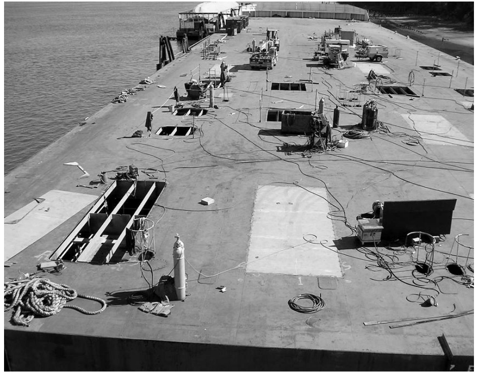
Workers at the Foss Rainier Shipyard installed 19 new deck plates on the Z Big 1 .
