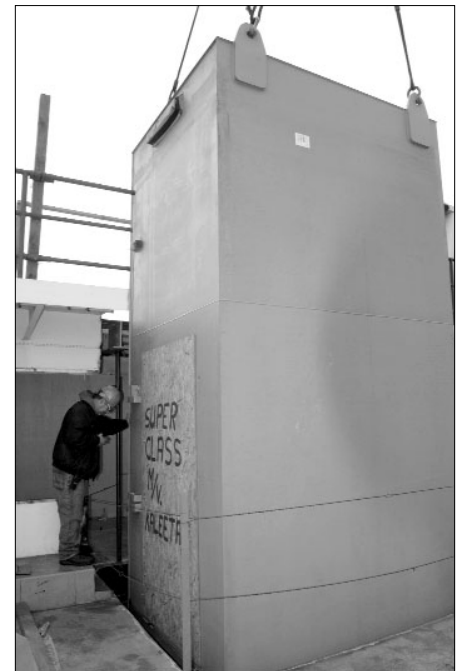
Rigger Foreman Jim Mosman radios instructions to Foss 300 operator John Tarabochia as the elevator shaft descends the last few feet into the ferry Kaleetan.
