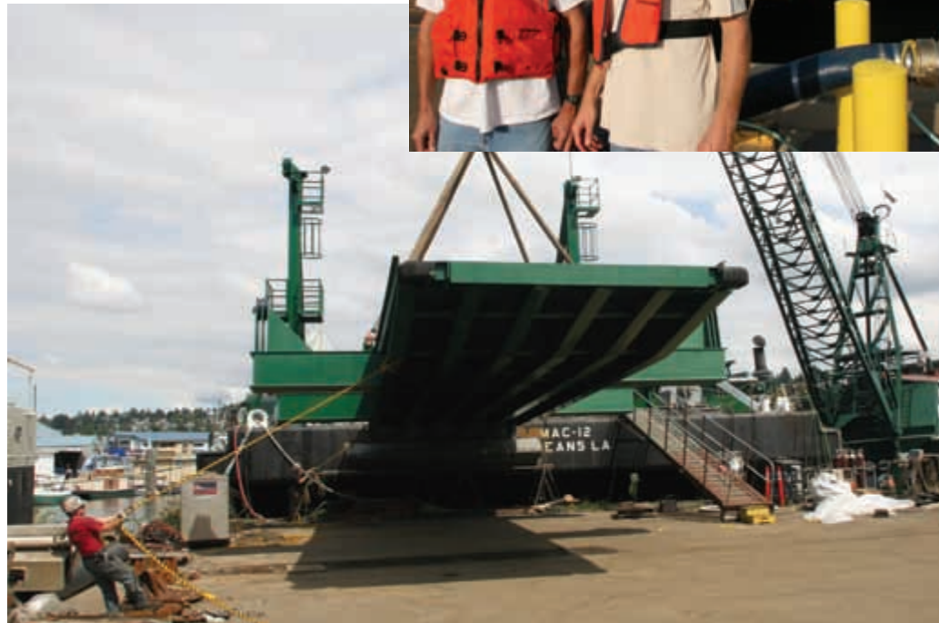
Jim Fox holds the tag line as the derrick Foss 300 lowers a new ramp into place on the barge Marmac 12 . The ramp measures 60-by-16 feet and weighs 44 tons.
