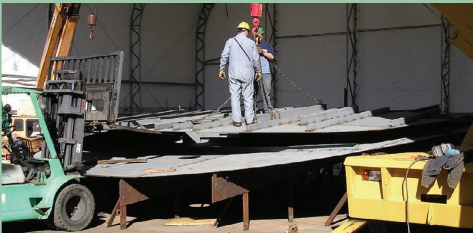
Foss Rainier Shipyard Yard Foreman Troy Schreiner , foreground and welder Brian Parsons ready a bow section bulkhead to be lifted into position for the hybrid-powered Dolphin tug now under construction. Not pictured is lead man Todd Hall , operating the crane.
