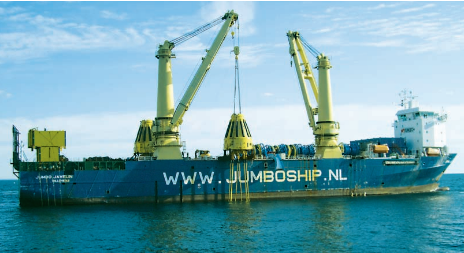
A subsurface buoy, to which LNG tankers will link and offload their cargo, is lowered from a heavy-lift ship into the Atlantic Ocean near Boston.
