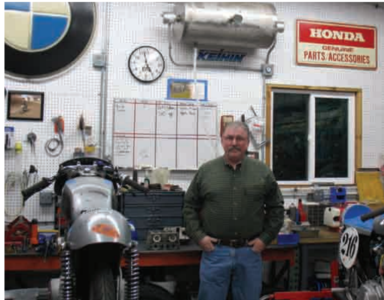
Mark Troutman built the hybrid system that heats his shop. Above his head is the storage tank for the heated water that circulates through the floor.
